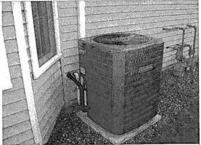
14. Model unit HVAC condenser
