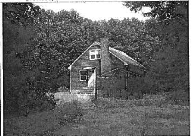
28. This old single-family house located at northeast corner of Property requires demolition, prior to developing the units planned for this location
