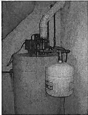
15. Model unit domestic hot water heater with associated thermal expansion tank
